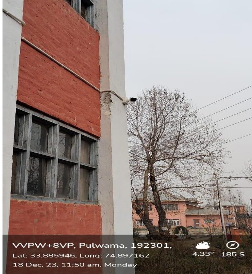
Campus under CCTV Surveillance
